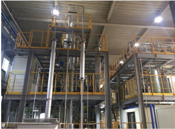
KCRC WASTE GAS CAPTURE PILOT PLANT
