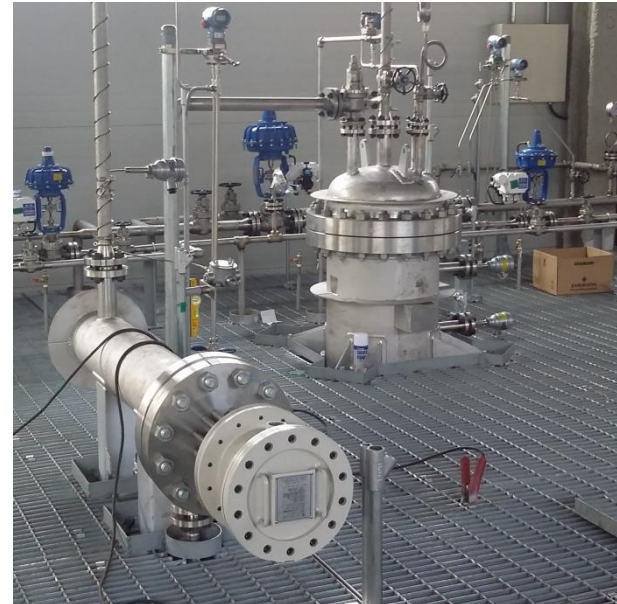
KIER WGS REACTION PILOT PLANT
